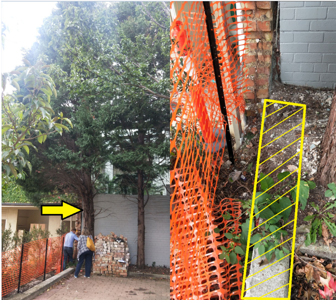
Figure 2. Tree to be removed marked by arrow, and concrete foundation marked in hatched area.
